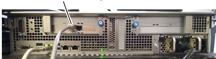
Ethernet cable in PCI NIC port 0
